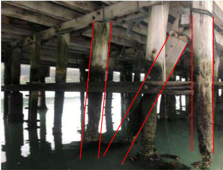
Photograph 3 – Bent 5, note broken raker pile and waisted vertical piles.
