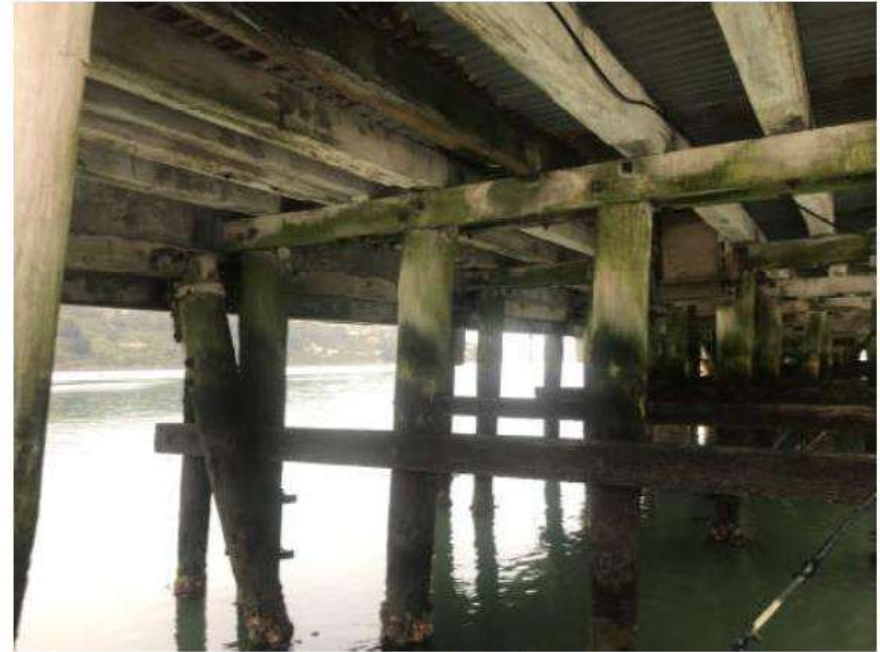
Photograph 2 – Underside of Wharf, note broken raker pile.
