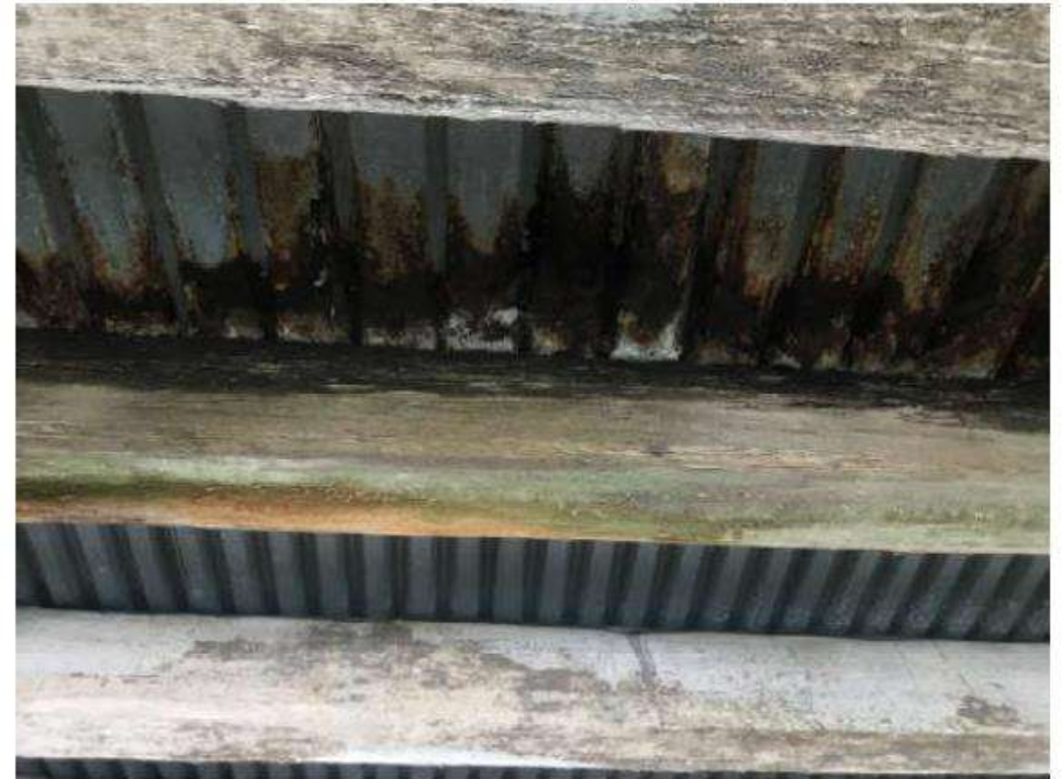
Photograph 4 – Underside of Wharf showing corrosion of the steel form.
